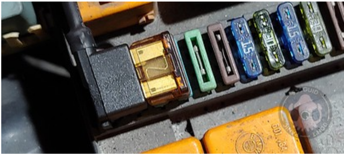
Figure 4. An example of an installed vampire fuse adapter.
